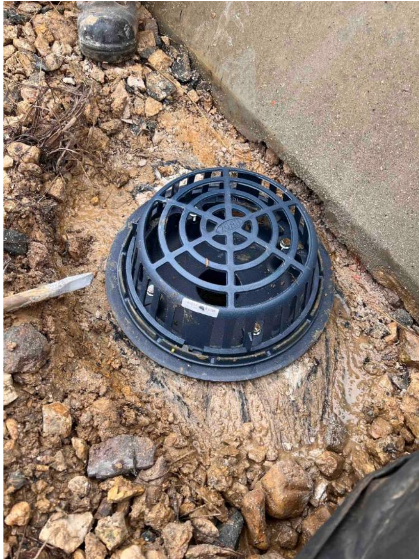
Drain Frame and Grate
