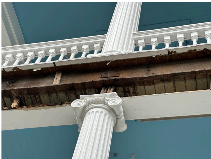
Second Floor porch - typical splits and buckling
