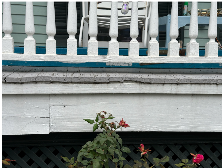
First Floor porch - typical splits and buckling
