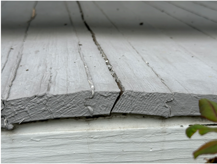
First Floor porch - typical splits and buckling
