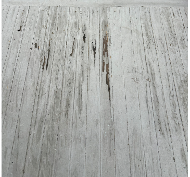
First Floor porch - typical condition of the boards paint peels off do to the dampness of the wood
